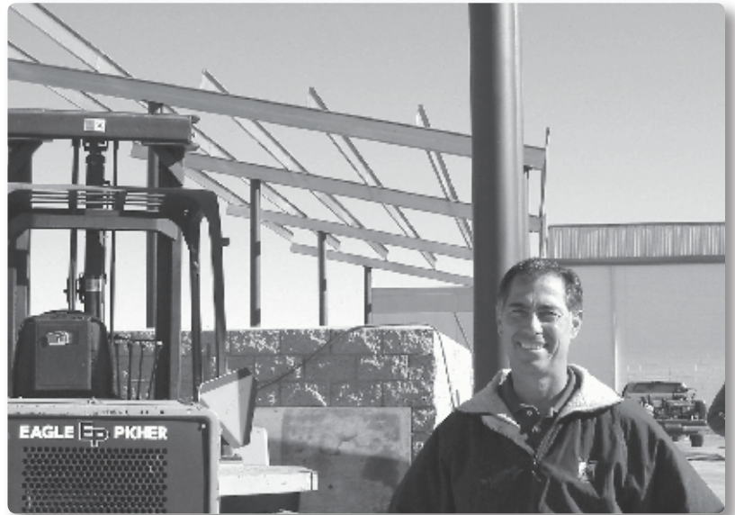
Jim Spallino, President of Great White Dental Lab, in front of the 100kW solar array under construction in the facility's parking lot.
